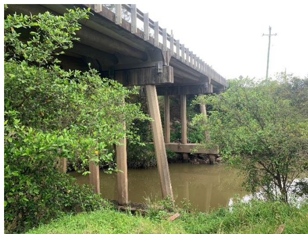
Looking south from the lower alluvial terrace on the northern creek bank (adjacent to BH2)
