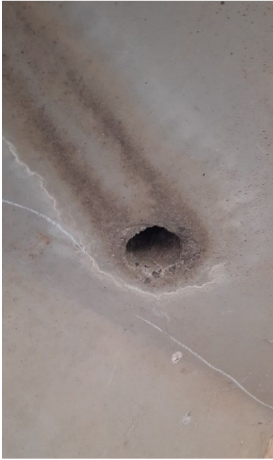
Plate 6.6 View of crevice in concrete underneath Spring Creek bridge
