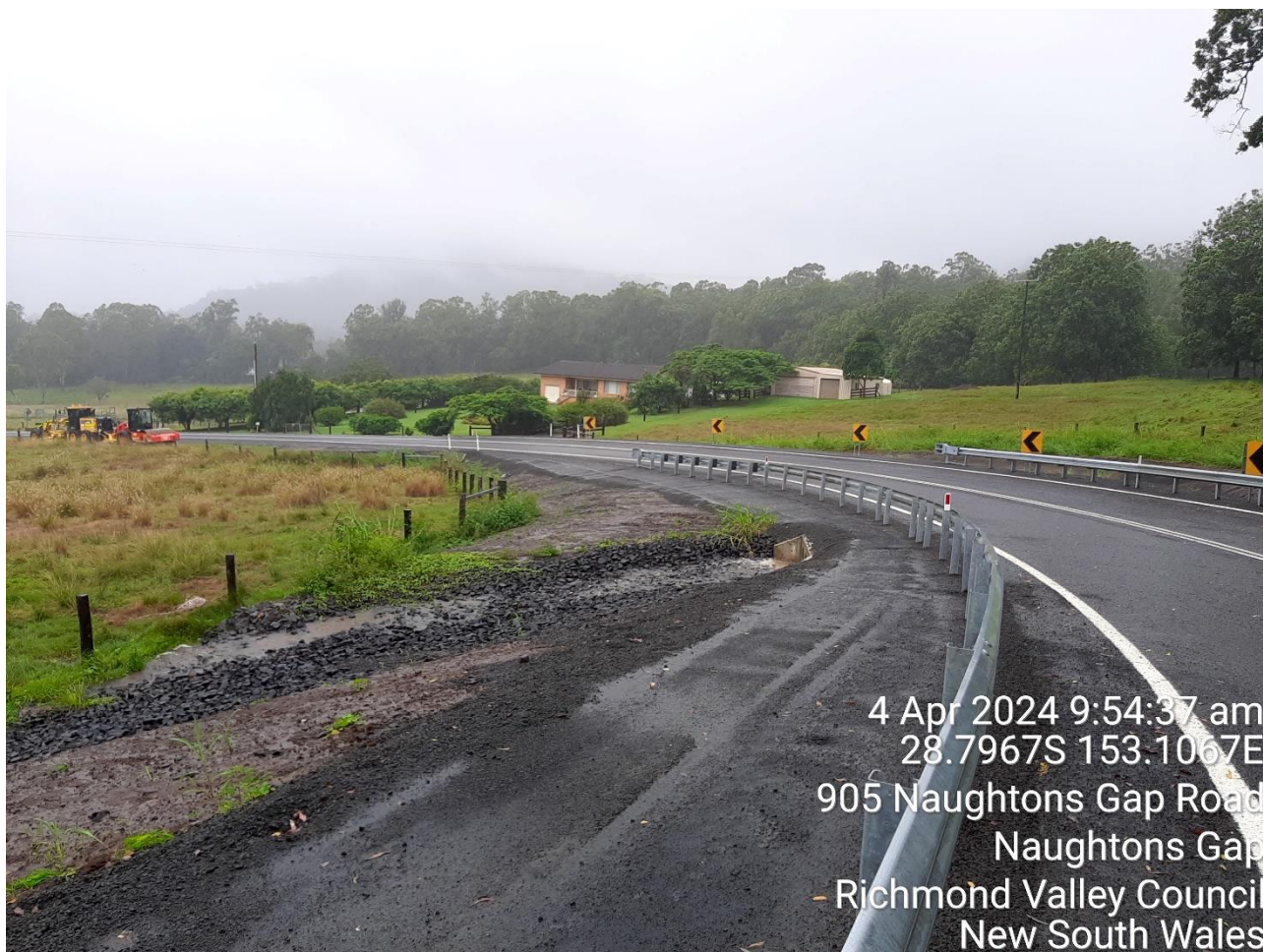
Image 2 – Photograph showing the constructed road widening, culvert and associated drainage impacting 925 Naughtons Gap Rd.
