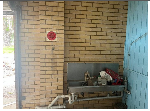
Photo 01. Chemicals stored within Building A
