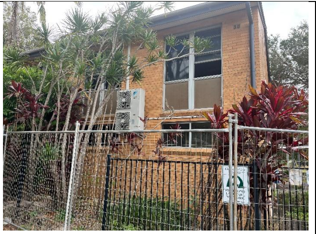
Photo 02. Refrigerant within AC unit Building A
