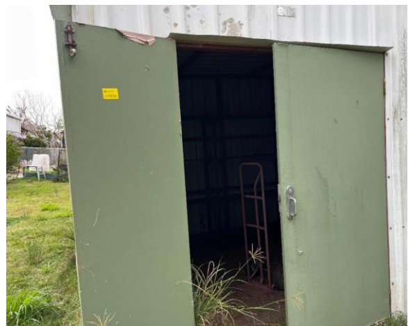
Line ID 37: External, Building C, Throughout, Doors, Green Paint - Lead Detected (0.12% w/w)
