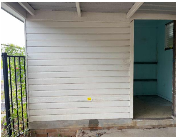
Line ID 11: External, Building B, Throughout, To Walls, Cream Paint (Coating Material) - No Asbestos Detected
