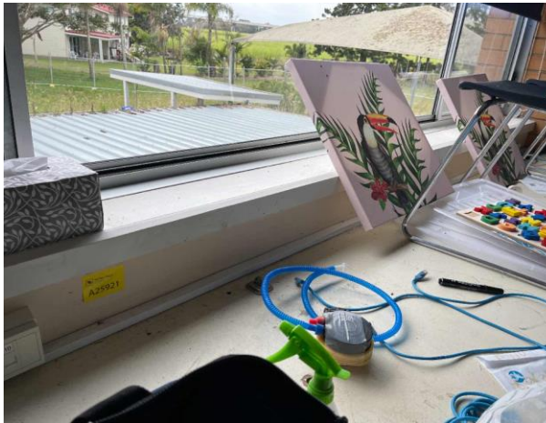
Line ID 25: Internal, Building A, Level 1, Enclosed Verandah, Northern and Western Infill Panels Below Windows, Compressed Cement Sheet - No Asbestos Detected
