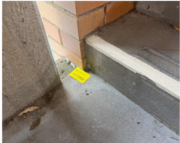
Line ID 2: External, Building A, Level 1, Stairs, To Floor, Mastic - Chrysotile Asbestos Detected
