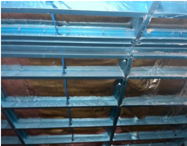
Line ID 58: Internal, Building E Ground Floor, Ceiling Space, Throughout, Sarking Insulation - Suspected SMF
