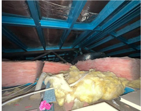
Line ID 57: Internal, Building E Ground Floor, Ceiling Space, Throughout, Loose Insulation - Suspected SMF
