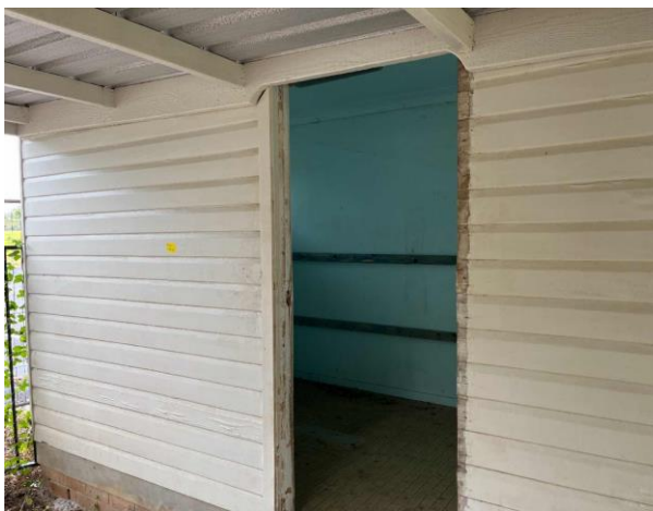
Line ID 36: External, Building B, Throughout, Walls, Eaves and Columns/Frame Work of Walkway, Cream Paint - Lead Detected (<0.005% w/w)
