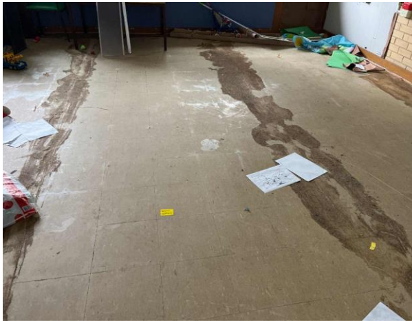
Line ID 27: Internal, Building A, Level 1, Throughout, Floor, Cream Vinyl Floor Tiles - Chrysotile Asbestos Detected
