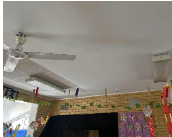
Line ID 26: Internal, Building A, Level 1, Throughout, Ceilings, Plaster Board - No Asbestos Detected
