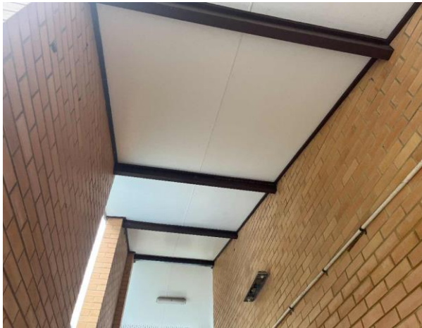
Line ID 1: External, Building A, Level 1, Stairs, Ceiling, Fibre Cement Sheet - Chrysotile Asbestos Detected
