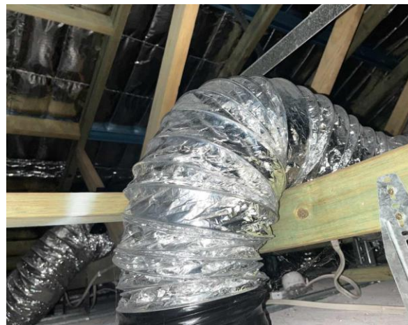
Line ID 49: Internal, Amenities Block, Ceiling Void, Flexible Air Conditioning Ductwork Throughout, Insulation Material - Suspected SMF
