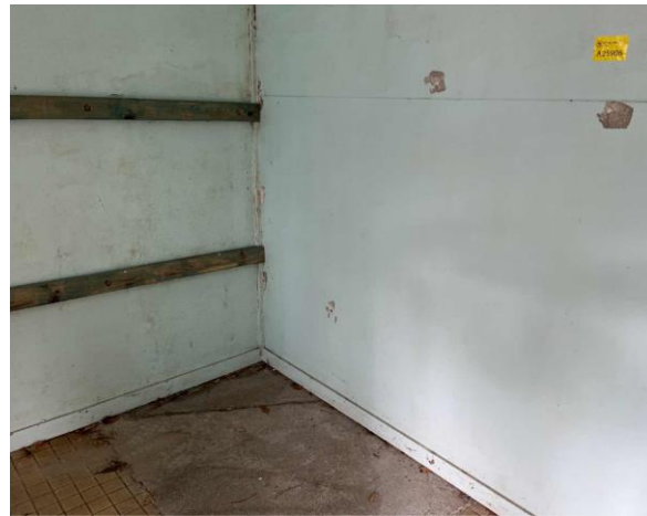
Line ID 31: Internal, Building B, Northern and Central Room, Walls (Excluding Center Wall Between Rooms), Fibre Cement Sheeting - No Asbestos Detected
