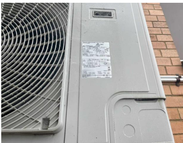
Line ID 63: External, Building A, Level 1, South Side, Daikin Air Conditioning unit, R410A Hydrofluorocarbon (HFC) - Non ODS Refrigerant
