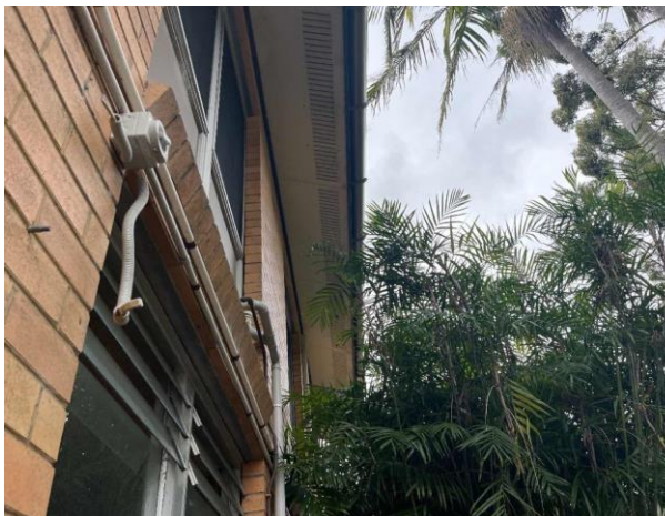
Line ID 3: External, Building A, Level 1, Throughout, Eaves, Fibre Cement Sheet - Chrysotile Asbestos Detected
