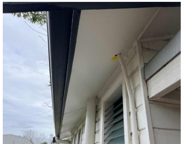
Line ID 10: External, Building B, Throughout, Eaves, Fibre Cement Sheetting - Chrysotile Asbestos Detected
