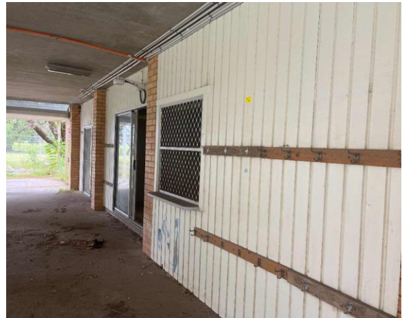
Line ID 33: External, Building A, Level 1, Throughout, Northern Walls, Cream Paint - Lead Detected (<0.005% w/w)
