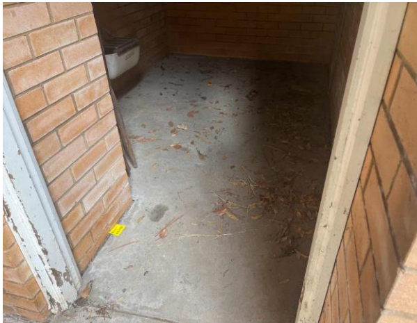
Line ID 21: Internal, Building A, Ground Floor, Storage Room Under Stairs, To Floor, Expansion Joint - Chrysotile Asbestos Detected
