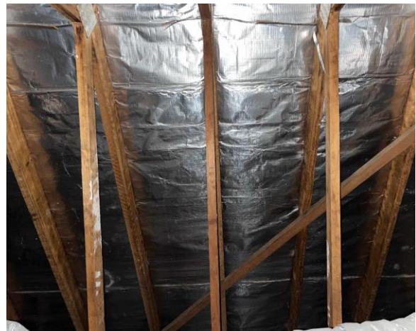
Line ID 55: Internal, Building A, Level 1, Ceiling Void, Throughout, Sarking Insulation - Suspected SMF
