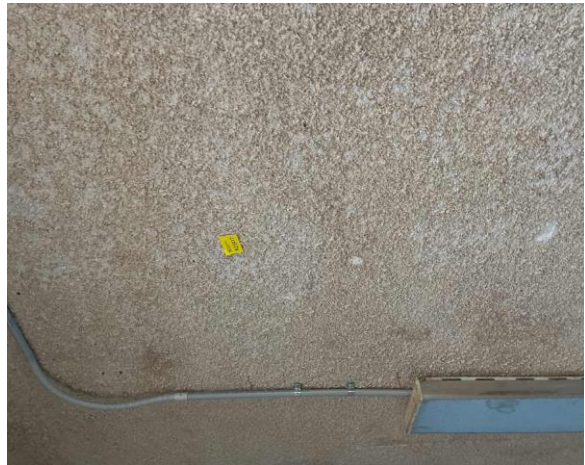
Line ID 22: Internal, Building A, Ground Floor, Throughout, Ceiling, Vermiculite - No Asbestos Detected
