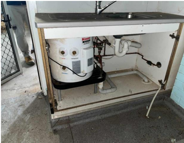
Line ID 52: Internal, Building A, Ground Floor, Canteen, Hot Water Heater Under Bench, Internal Insulation - Suspected SMF
