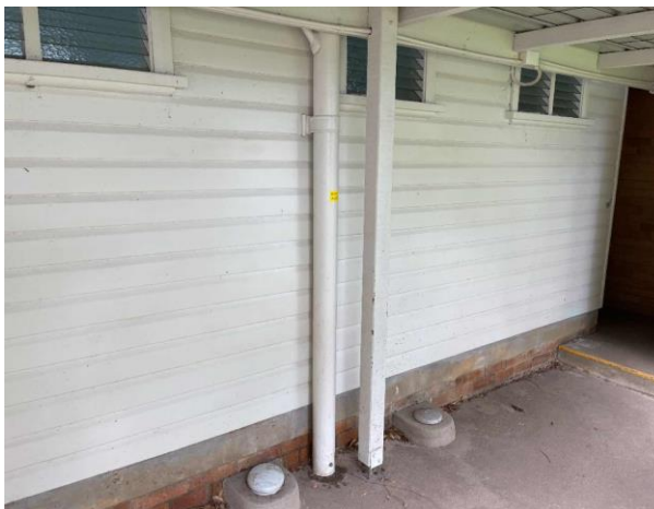
Line ID 9: External, Building B, Throughout, Down Pipe to Western Wall, Moulded Fibre Cement - Chrysotile Asbestos Detected
