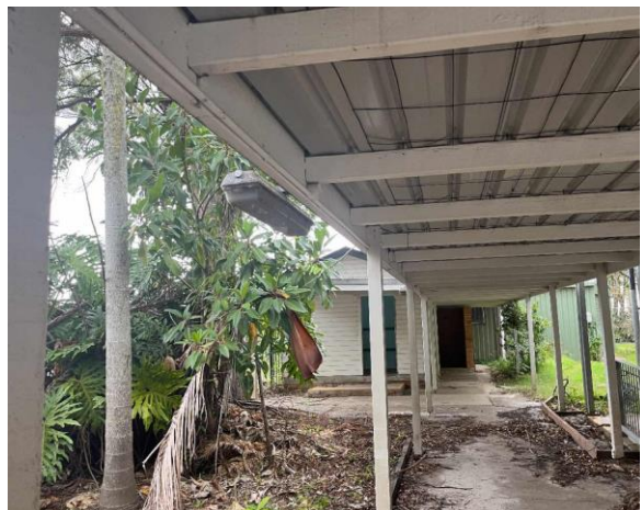
Line ID 60: External, Throughout, Throughout, Light Fittings, Ballast(s) - Suspected PCB
