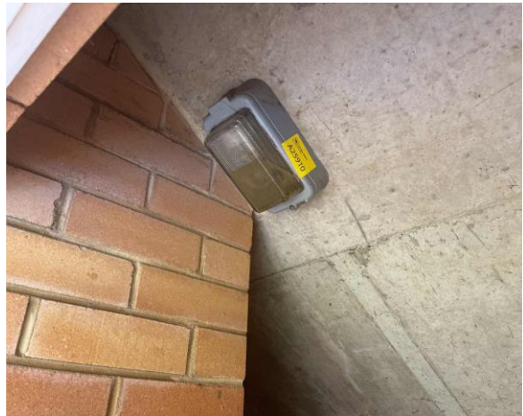
Line ID 20: Internal, Building A, Ground Floor, Storage Room Under Stairs, Between Metal and Glass of Wilco Light, Mastic - Chrysotile Asbestos Detected
