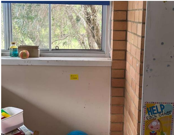
Line ID 44: Internal, Building A, Level 1, Enclosed Verandah, Infill Panels and Trim, Beige Paint - Lead Detected (<0.005% w/w)
