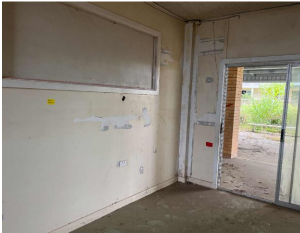
Line ID 19: Internal, Building A, Ground Floor, Eastern Room, Northern and Western Walls, Fibre Cement Sheet - No Asbestos Detected
