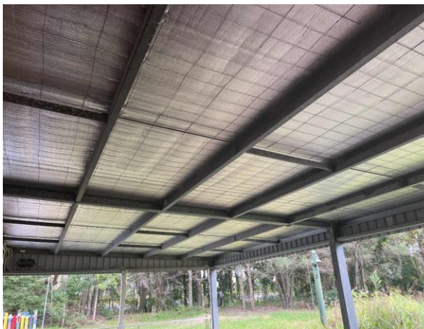
Line ID 48: External, Building A, Ground Floor, Covered Area, To Ceiling, Sarking Insulation - Suspected SMF
