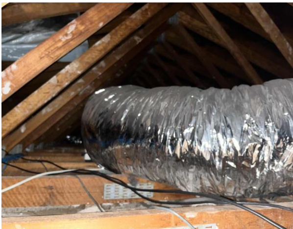
Line ID 54: Internal, Building A, Level 1, Ceiling Void, Flexible Air Conditioning Ductwork Throughout, Internal Insulation - Suspected SMF
