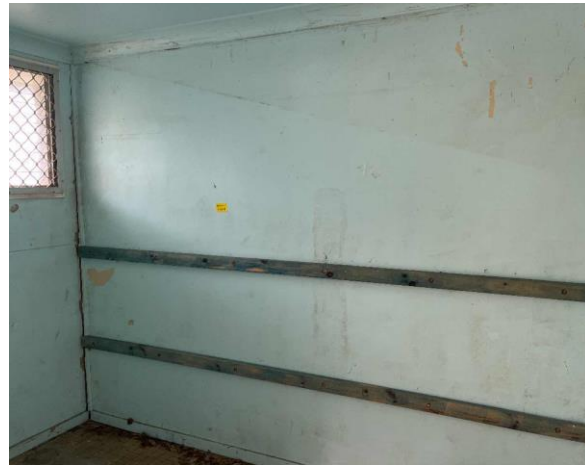
Line ID 45: Internal, Building B, Northern and Central Room, Walls and Ceiling, Blue Paint - Lead Detected (0.061% w/w)
