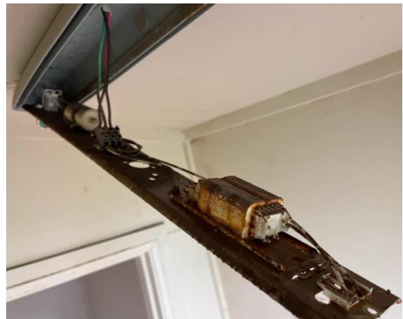
Line ID 62: Internal, Building B, Toilet Rooms, Ceiling, Capacitor(s) - Suspected PCB
