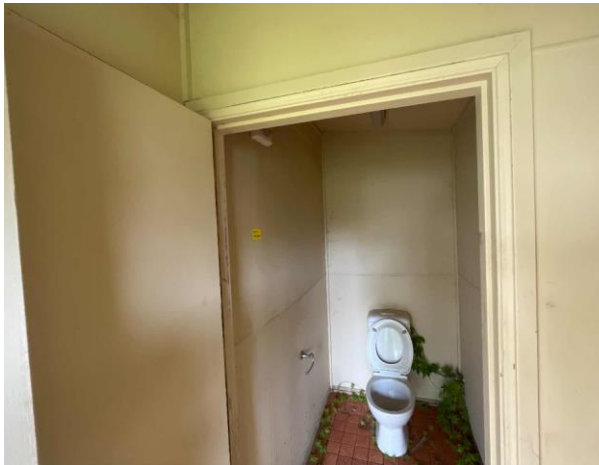
Line ID 32: Internal, Building B, Toilet Rooms, Walls And Ceilings, Fibre Cement Sheetting - No Asbestos Detected
