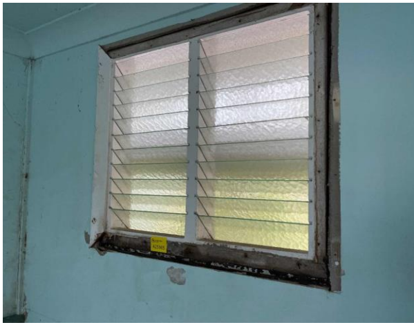
Line ID 30: Internal, Building B, Northern and Central Room, Mastic Between Wooden Pieces of Window Frame, Mastic Sealant - No Asbestos Detected
