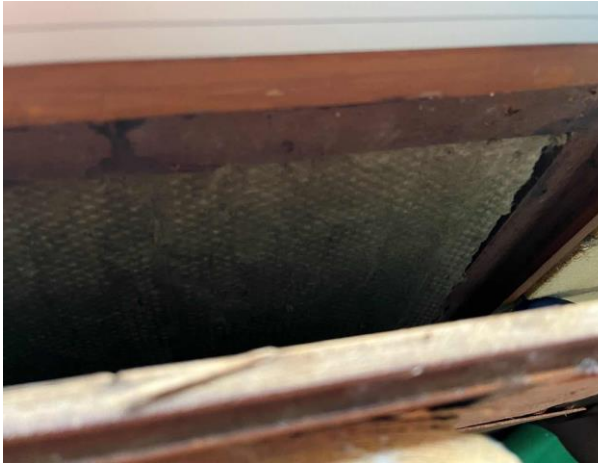
Line ID 56: Internal, Building A, Level 1, Throughout, Southern Wall, Behind Wooden Panels, Below Windows, Insulation Material - Suspected SMF
