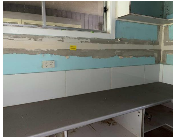
Line ID 16: Internal, Building A, Ground Floor, Canteen, North, East and South Walls, Fibre Cement Sheet - No Asbestos Detected
