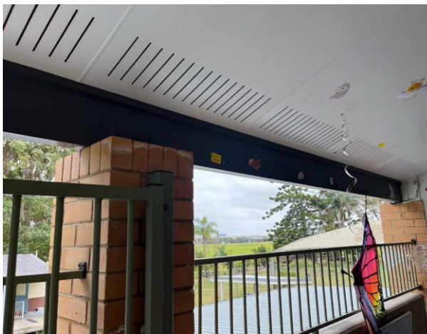
Line ID 34: External, Building A, Level 1, Verandah, Beams and Trim, Dark Grey Paint - Lead Detected (0.03% w/w)
