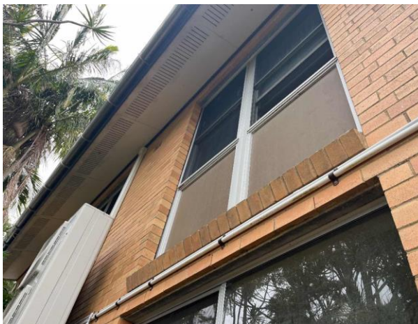
Line ID 5: External, Building A, Level 1, Throughout, Infill Panels, Below Windows, Compressed Cement Sheeting - Chrysotile Asbestos Detected
