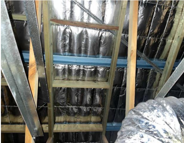
Line ID 50: Internal, Amenities Block, Ceiling Void, Throughout, Sarking Insulation - Suspected SMF
