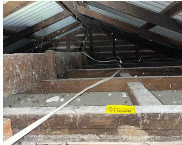
Line ID 47: Internal, Building B, Ceiling Space, Throughout, Dust - Lead Detected (330mg/kg)
