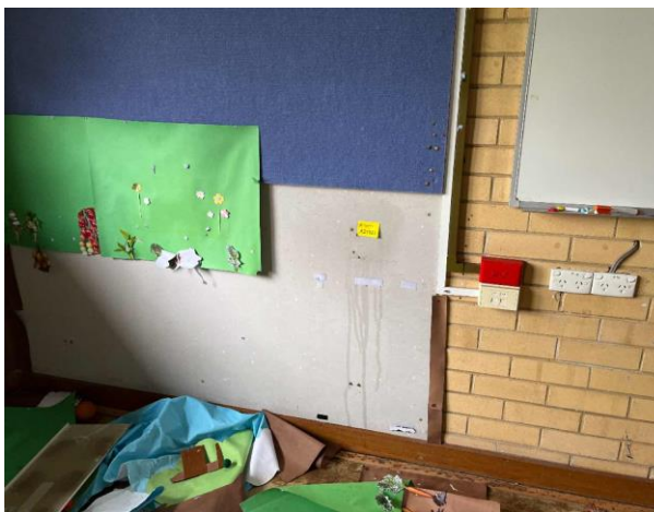
Line ID 23: Internal, Building A, Level 1, Class Room, South West Corner, Infill Panel, Fibre Cement Sheet - No Asbestos Detected
