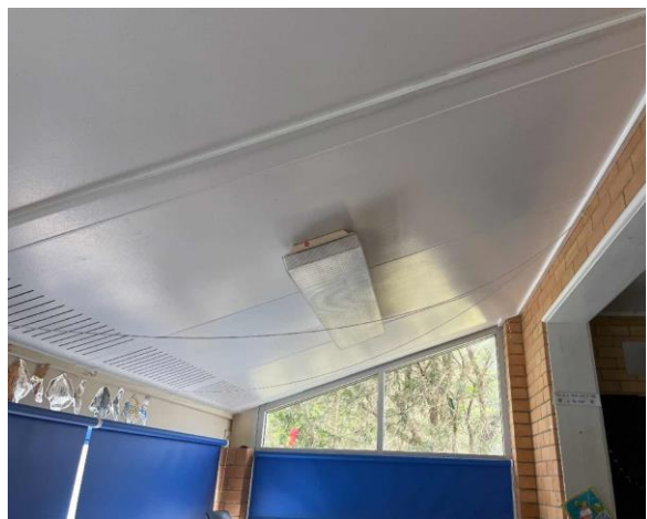
Line ID 24: Internal, Building A, Level 1, Enclosed Verandah, Ceiling, Fibre Cement Sheet - Chrysotile Asbestos Detected
