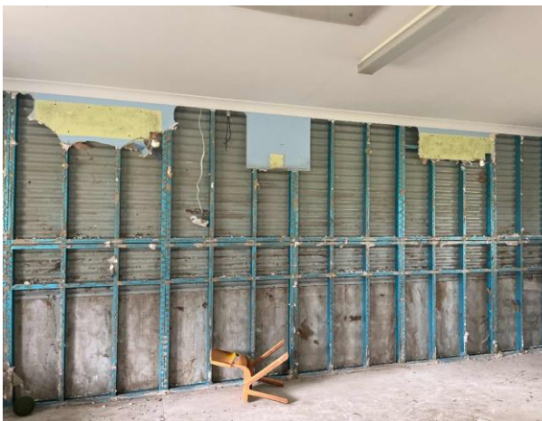
Line ID 59.1: Internal, Building E Ground Floor, West side, Behind Remanding Wall, Insulation Batts - Suspected SMF
