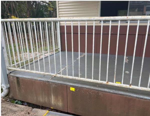
Line ID 13: External, Building E, Throughout, Lower 1/3 of Walls, Compressed Cement Sheet - No Asbestos Detected
