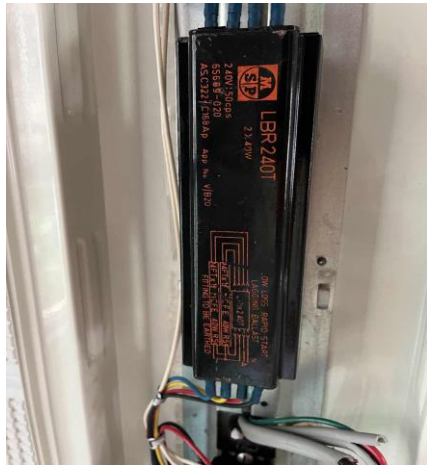
Line ID 61: Internal, Building A, Level 1, Throughout, Light Fittings, Ballast(s) - Suspected PCB
