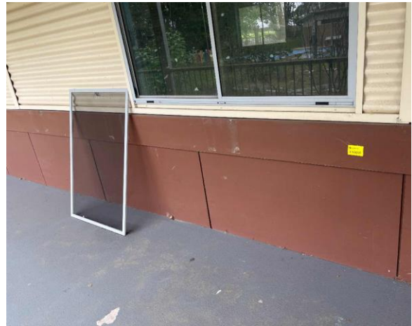
Line ID 39: External, Building E, Throughout, Lower Walls, Brown Paint - Lead Detected (0.01% w/w)
