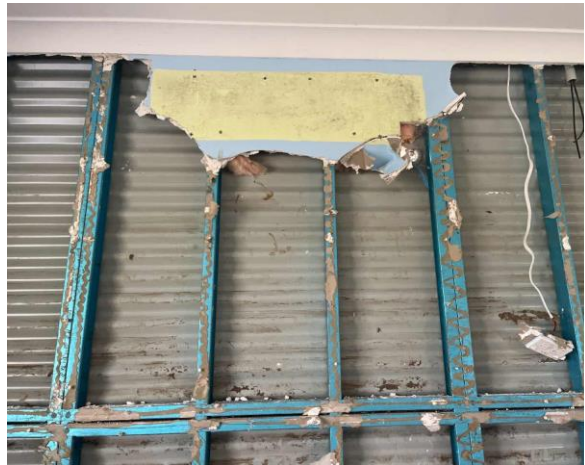
Line ID 59: Internal, Building E Ground Floor, West side, Behind Remanding Wall, Insulation Batts - Suspected SMF
