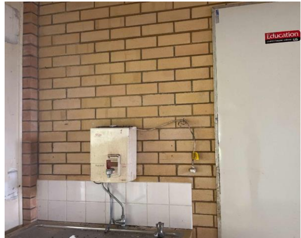
Line ID 53: Internal, Building A, Ground Floor, Eastern Room, Hot Water Boiler, Above Sink, Internal Insulation - Suspected SMF
