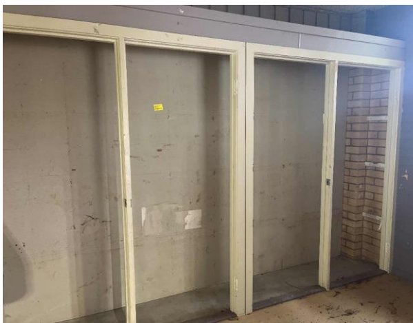
Line ID 17: Internal, Building A, Ground Floor, Central Room, Internal and External Walls of Cupboards, Fibre Cement Sheet - No Asbestos Detected
