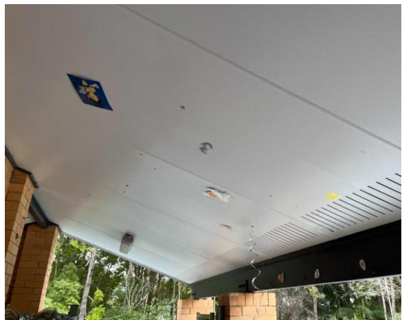
Line ID 6: External, Building A, Level 1, Verandah, Ceiling, Fibre Cement Sheet - Chrysotile Asbestos Detected
