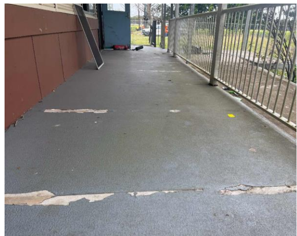
Line ID 12: External, Building E, South Side, Verandah Floor, Compressed Cement Sheet - No Asbestos Detected
