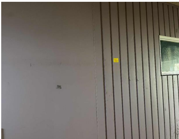
Line ID 42: Internal, Building A, Ground Floor, Central Room, Walls, Purple Paint - Lead Detected (<0.005% w/w)
