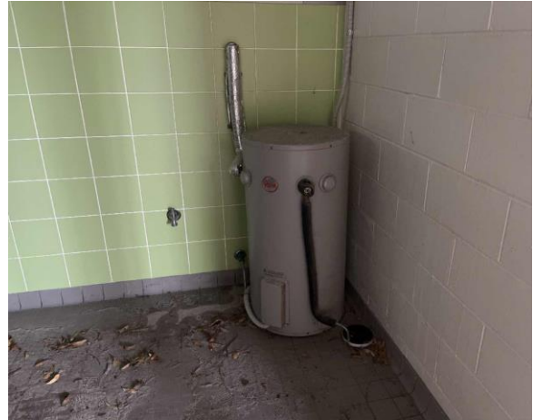
Line ID 51: Internal, Amenities Block, Female Ambulant Toilets, Within Hot Water Heater, Internal Insulation - Suspected SMF
