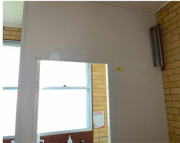
Line ID 29: Internal, Building A, Level 1, Toilet, South West Walls, Fibre Cement Sheet - No Asbestos Detected
