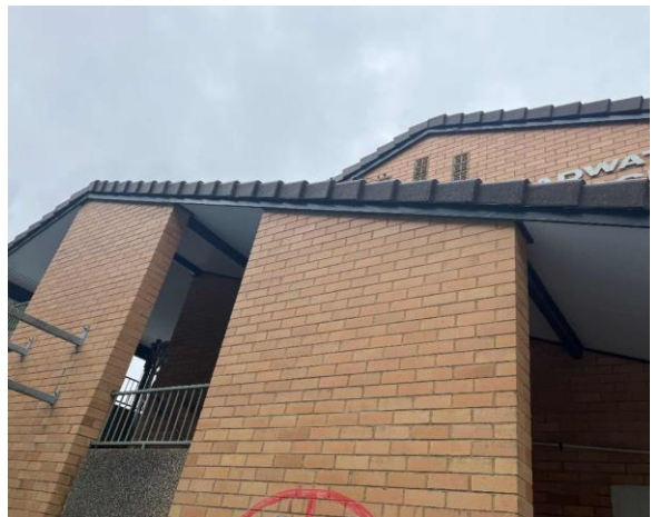
Line ID 4: External, Building A, Level 1, Throughout, Gable Verge Lining, Fibre Cement Sheet - Suspected Asbestos
