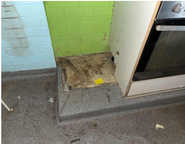
Line ID 15: Internal, Building A, Ground Floor, Canteen, Floor, Under Cabinets, Beige Vinyl Sheet - No Asbestos Detected
