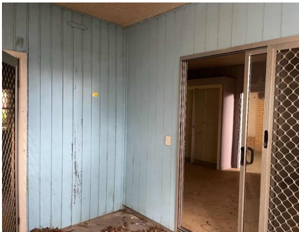
Line ID 40: Internal, Building A, Ground Floor, Bubler Room, Walls, Blue (Light) Paint - Lead Detected (<0.005% w/w)
