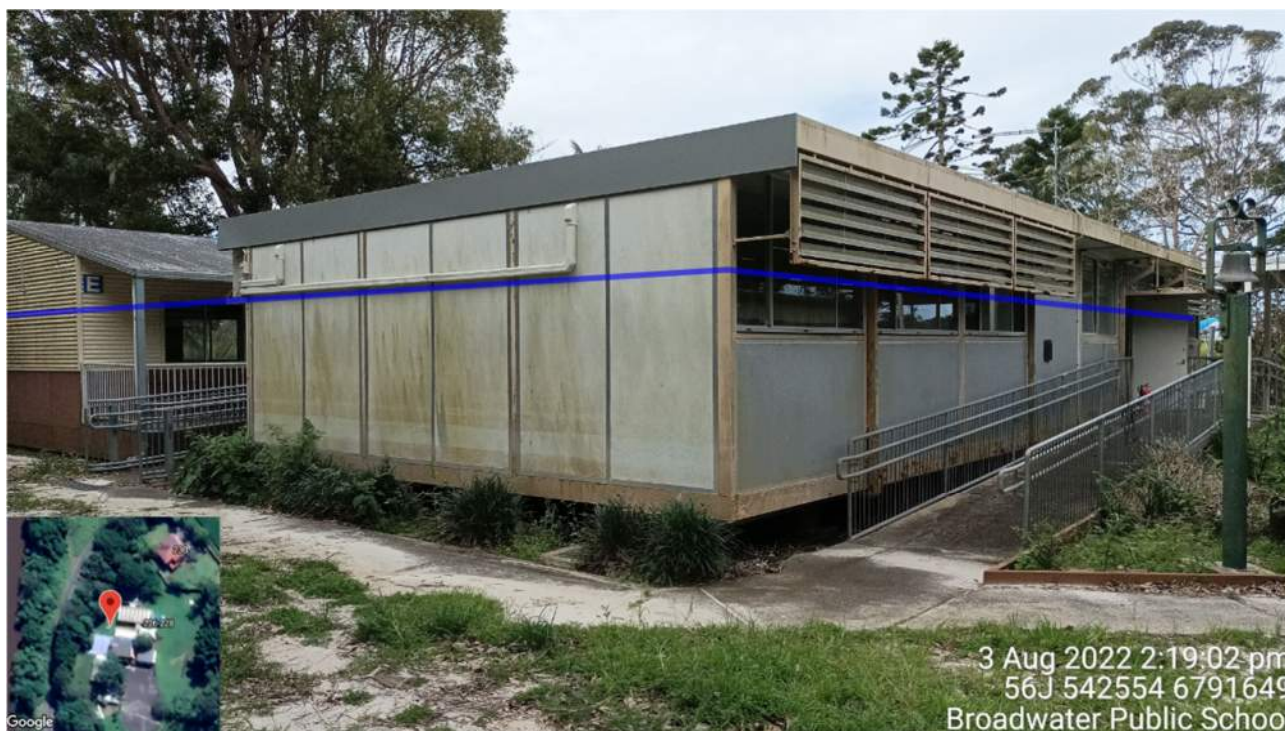
Plate 4-2 March 2022 approximate peak flood level at Block D11066 (Learning Space) denoted by blue line
