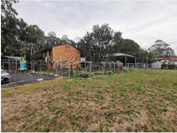
Photograph 1: Unoccupied, flood damaged buildings barricaded with chain link fencing
