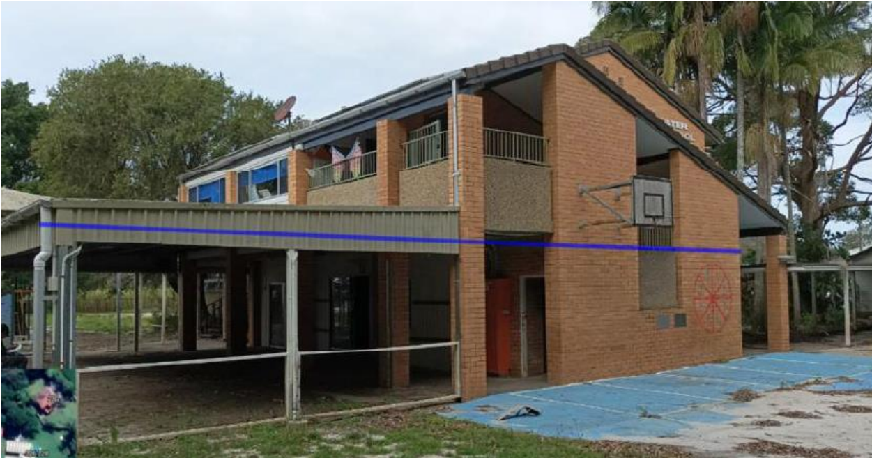
Figure 25: Building A – with Feb 2022 flood height indicated by blue line (Source: Acor Consultants)
