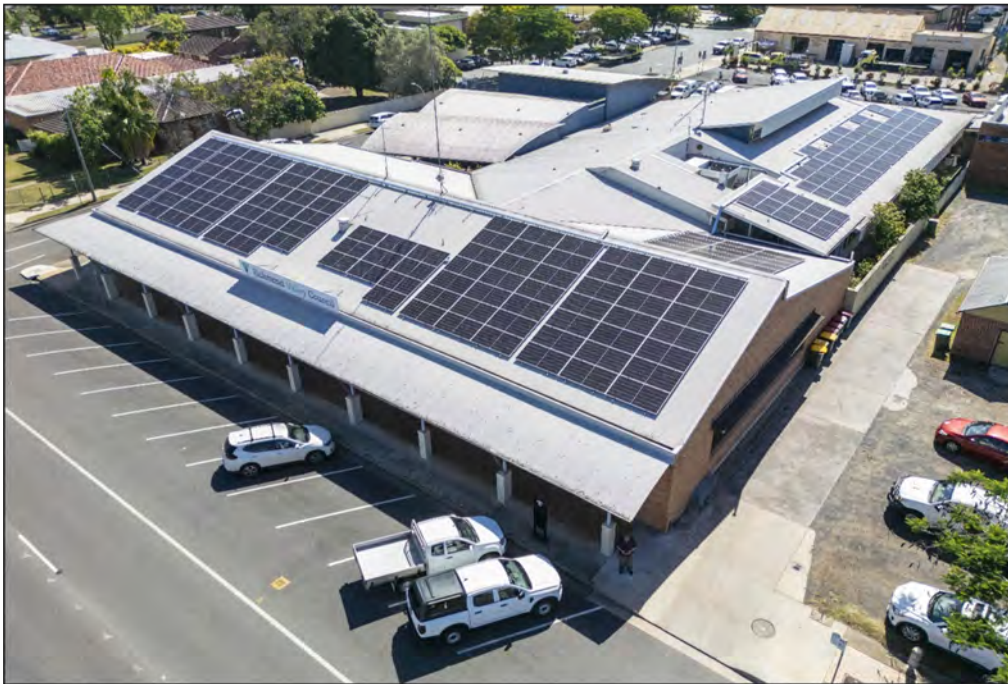
View via drone of the new solar panels on the Council administration building in Casino
