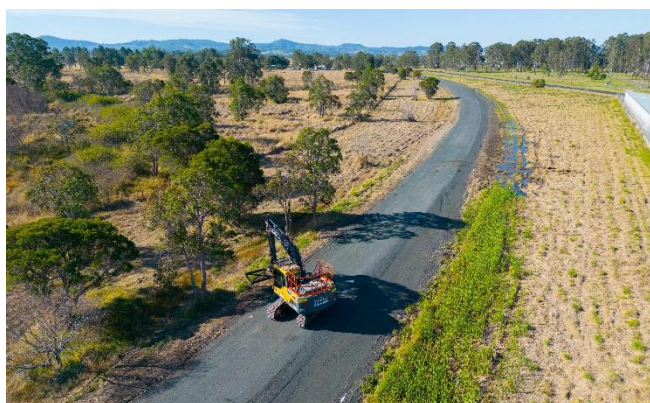
Work is nearing completion on the Casino-Bentley section of the Northern Rivers Rail Trail.
