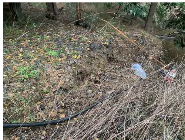
Looking west at the landslide, showing fill mixed with alluvial sands exposed along the slip.
