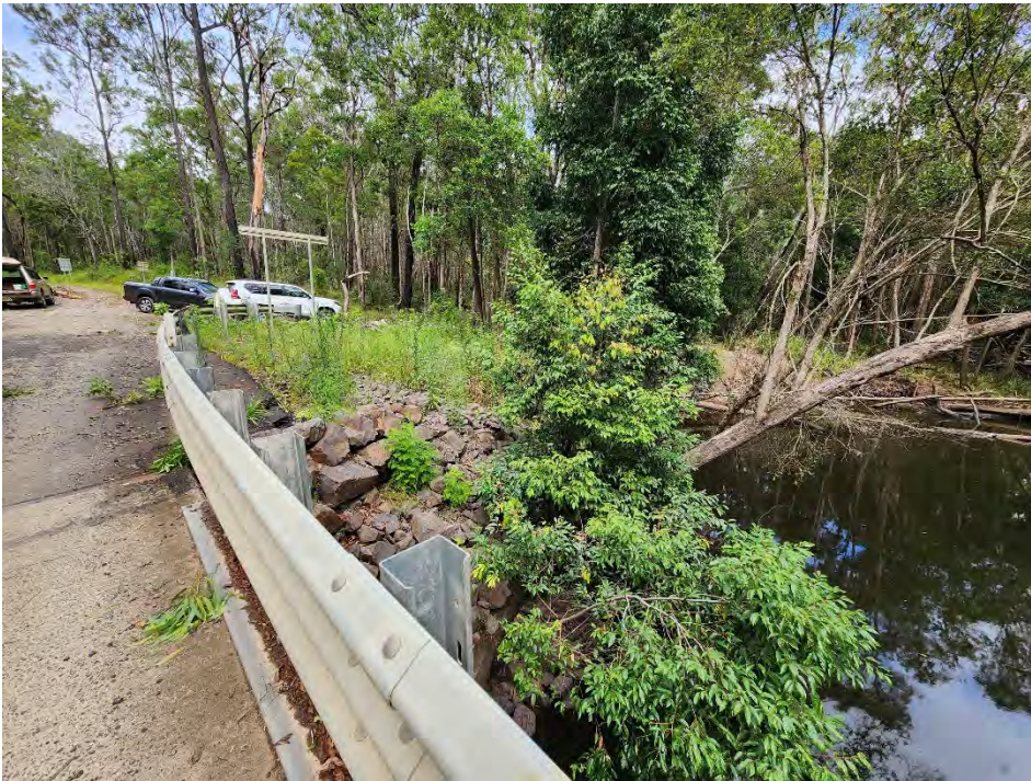
Plate 6 – Photo showing southern creek bank with signs of erosion and scour. Scour rock has been placed to reduce erosion.
