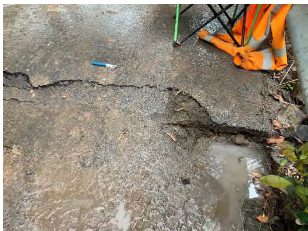
Differential movement between the bridge deck and the northern abutment pavement
