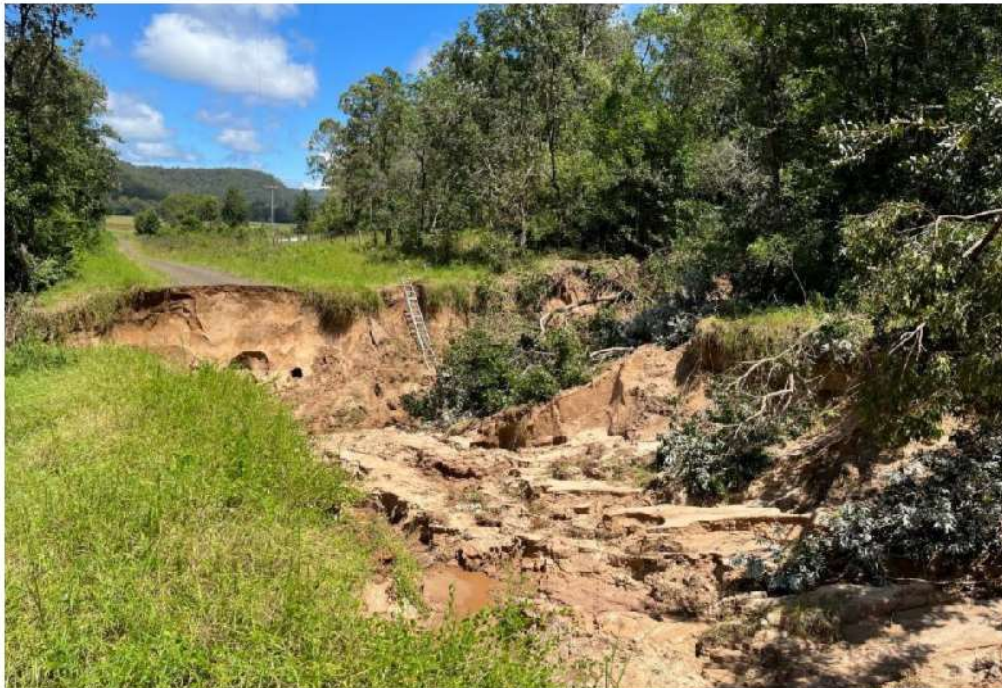
Council is facing more than $100m in major road repairs following the floods. This washaway on Upper Cherry Tree Rd, Mongogarie left residents isolated.
