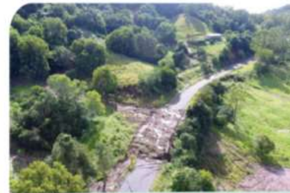
Naughtons Gap Road landslip
