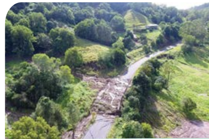
Naughtons Gap Road landslip
