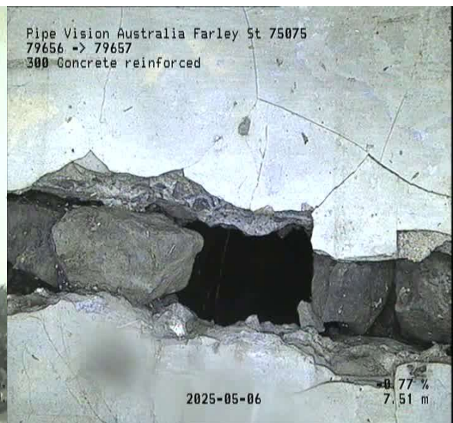
Image 2 – Stormwater pipe with poor structural score with good good service score – eg structure damaged can convey stormwater.
